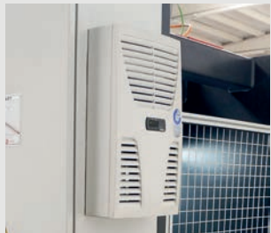
Electrical Cabinet Cooling System
